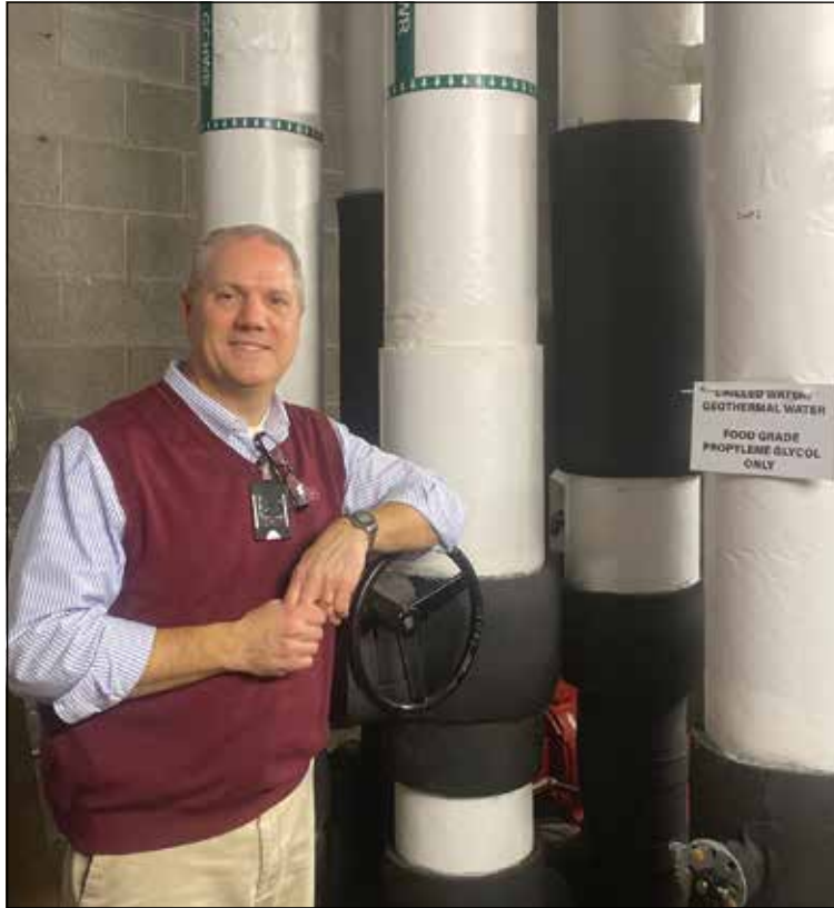
Kevin Davis, assistant principal at Johnson Senior High School, stands next to the new geothermal HVAC system in the school's basement. Photo by George Zan.
