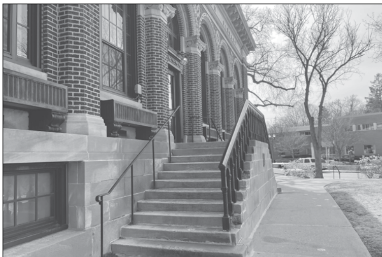
Entrances at the St. Anthony Park Branch Library are among items that will be repaired while the building is closed for several weeks until sometime in June. Photos by Janet Wight.
