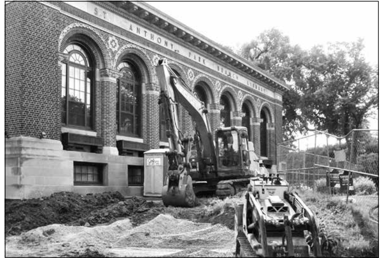
Heavy equipment has dug up the grounds around the St. Anthony Park Branch Library as the facility undergoes repairs and maintenance work. Photo by Kathy Henderson.
