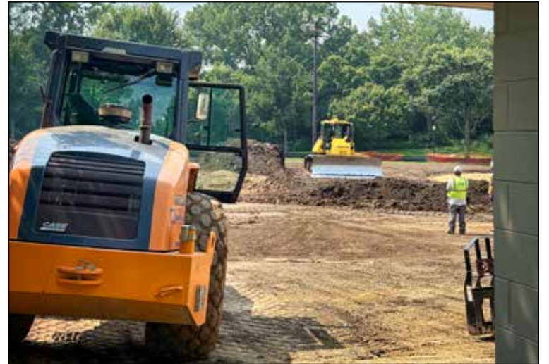
Construction crews and earth-moving machinery are a common site at Langford Park as it undergoes a major facelift. Photo by Bill Brady.
